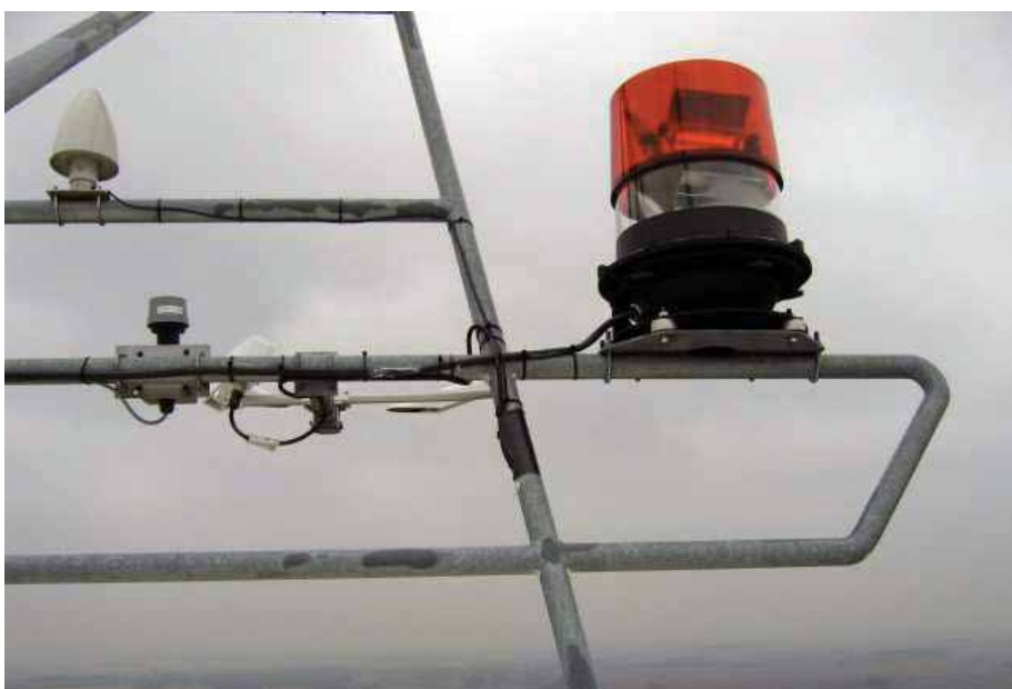
Figure 4. The Vaisala PWD20W installed on a wind turbine in the recommended location below the obstruction light on the nacelle.
